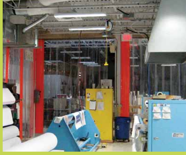
Portland Color made many green changes to its facilities, including the fabric print room. The room has an extra-large vent on both the printer and the heat transfer equipment. The disk on the ceiling behind the light is part of the humidification system the company installed to maintain even humidity year round. Photo: Portland Color.
